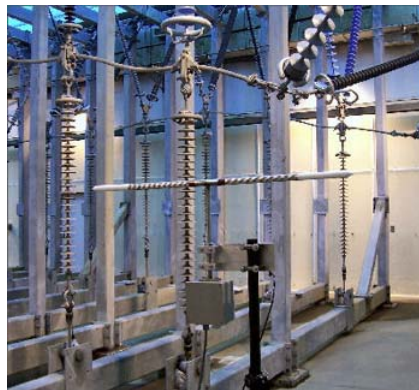
TRM operating in 10 kV/m electric field.
